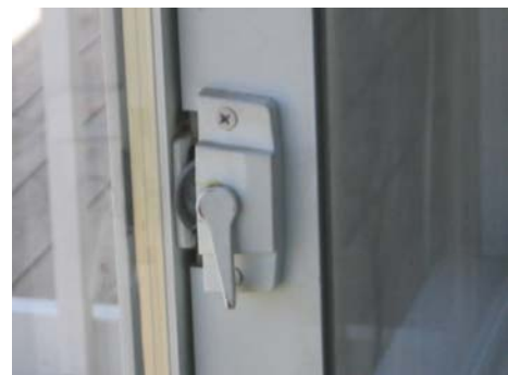
WINDOW LOCK DEFECTIVE AT MASTER BEDROOM WEST WALL
