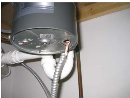
EXPOSED HIGH VOLTAGE AT SINK DISPOSAL
