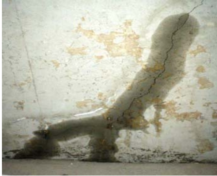
ACTIVE WATER INFILTRATION AT SOUTH FOUNDATION WALL CRACK
