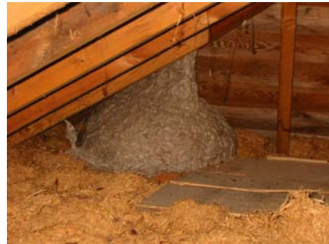
LARGE HORNETS NEST LOCATED IN ATTIC
