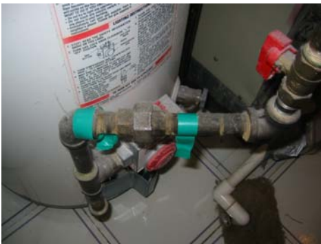
GAS LEAKS DETECTED AT UNION ON SUPPLY LINE SERVICING WATER WATER
