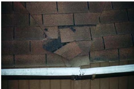
ROOF SHINGLES DAMAGED AT GARAGE REAR ELEVATION
